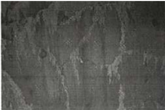
Figure 2. Leaching of \text{Ca}(\text{OH})_2 from concrete as a result of water filtration.
